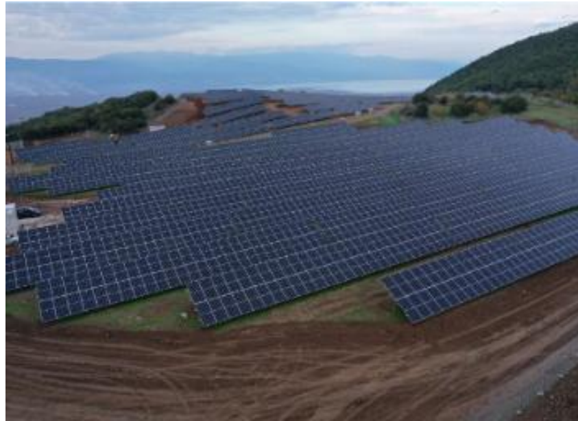
PV system of 999.9 kWp in Lamia, Fthiotida Prefecture
